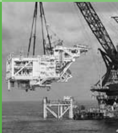
Left: Wellhead platform construction, Bayu-Undan liquids project, Timor Sea. Photograph courtesy of ConocoPhillips Australia Pty Ltd.
