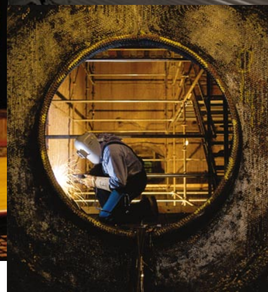
Welders at the AmerenCIPS Coffeen Plant overhaul a boiler as part of a 1997 plant outage that required 28% fewer manhours than earlier outages.
