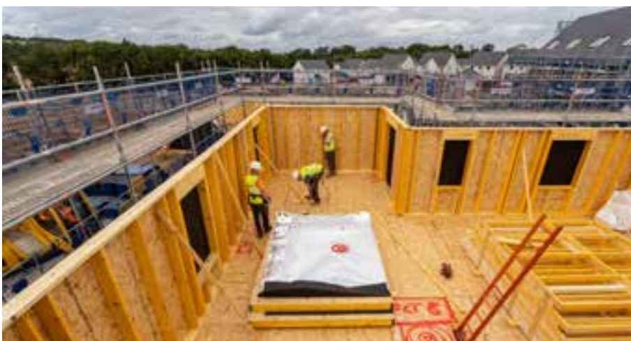
← Above and left: Oregon timber frame installation at Heritage Grange, Edinburgh, Scotland.
