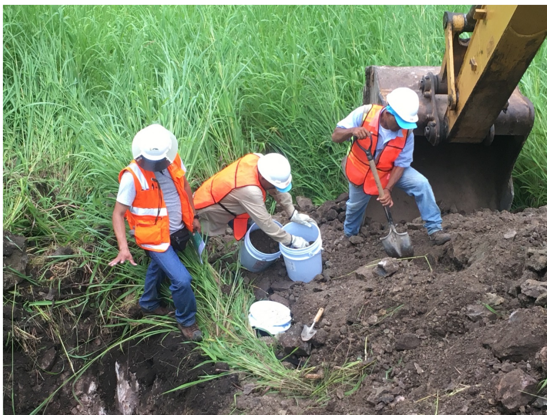
TSF ground Investigation test pit LIPT042 on the northern drainage channel above the main dam.
