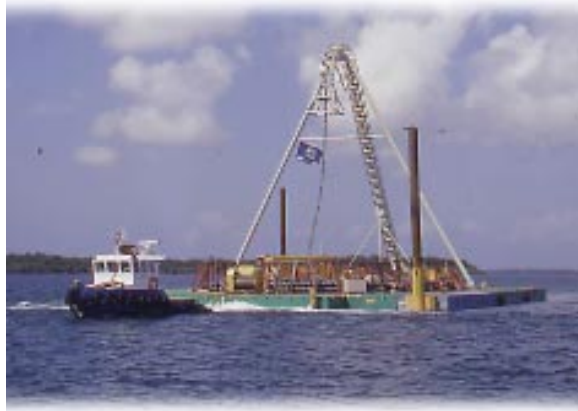
CUC's looped T&D system project continued with the laying of 14 miles of 69KV transmission submarine cable across the North Sound in May 2001. The barge above laid cable in connection with the eastern loop scheduled for completion in late 2002.
