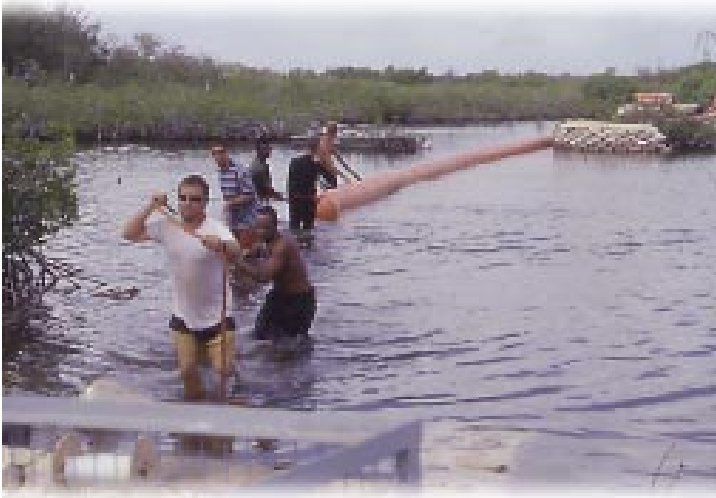
Employees of ABB T&D Power Company, Inc. and its subcontractors contribute to the submarine cable-laying project by carefully guiding the cable through a designated environmental zone near Cayman Kai. Outcroppings of mangrove were sandbagged for extra protection.
