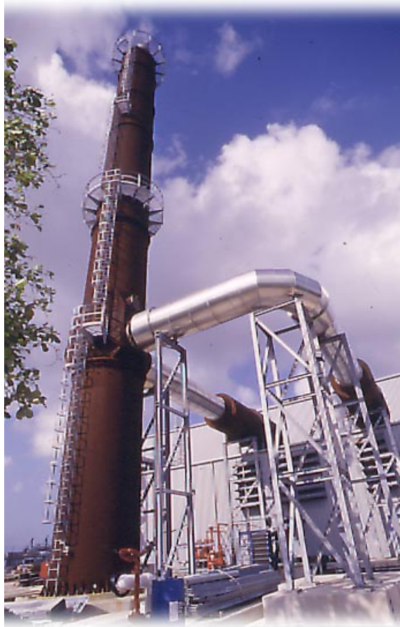
CUC installed a 140-foot exhaust stack to the engine room housing its two MAN B&W generating units. This stack will improve air quality surrounding the plant.
