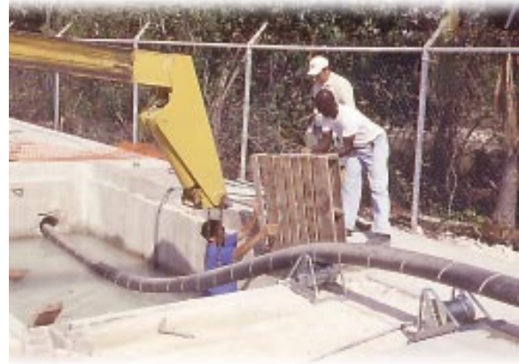
Work is progressing at the Morgan's Harbour/West Bay landing of the 69KV transmission submarine cable project. This landing comprises part of the western loop expected to be completed in October 2001.
