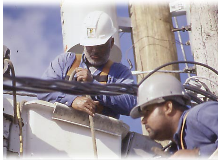
Lineman Foremen Clinton Stewartson and Johnny Ebanks, perform upgrades on de-energised and grounded lines in helping CUC provide world-class, reliable service to its customers.
