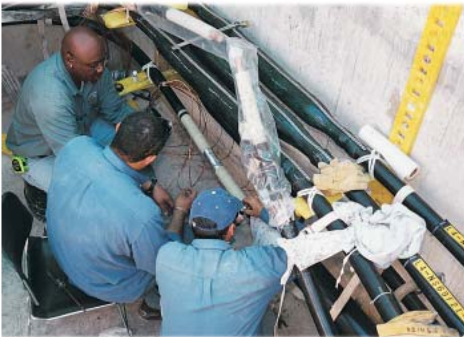
Albert McLean, Lineman Foreman, Thomas Ebanks, Industrial Electrician, and Harold Rivers, Lineman Apprentice, install splices to connect sections of the 69KV underground cable. This cable is part of the transmission loop which will enhance the reliability of service to our customers.
