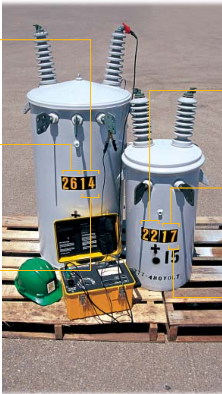
CUC has over 3,940 transformers installed on its distribution lines. These transformers are used to step down higher distribution voltage to levels usable by our customers.
