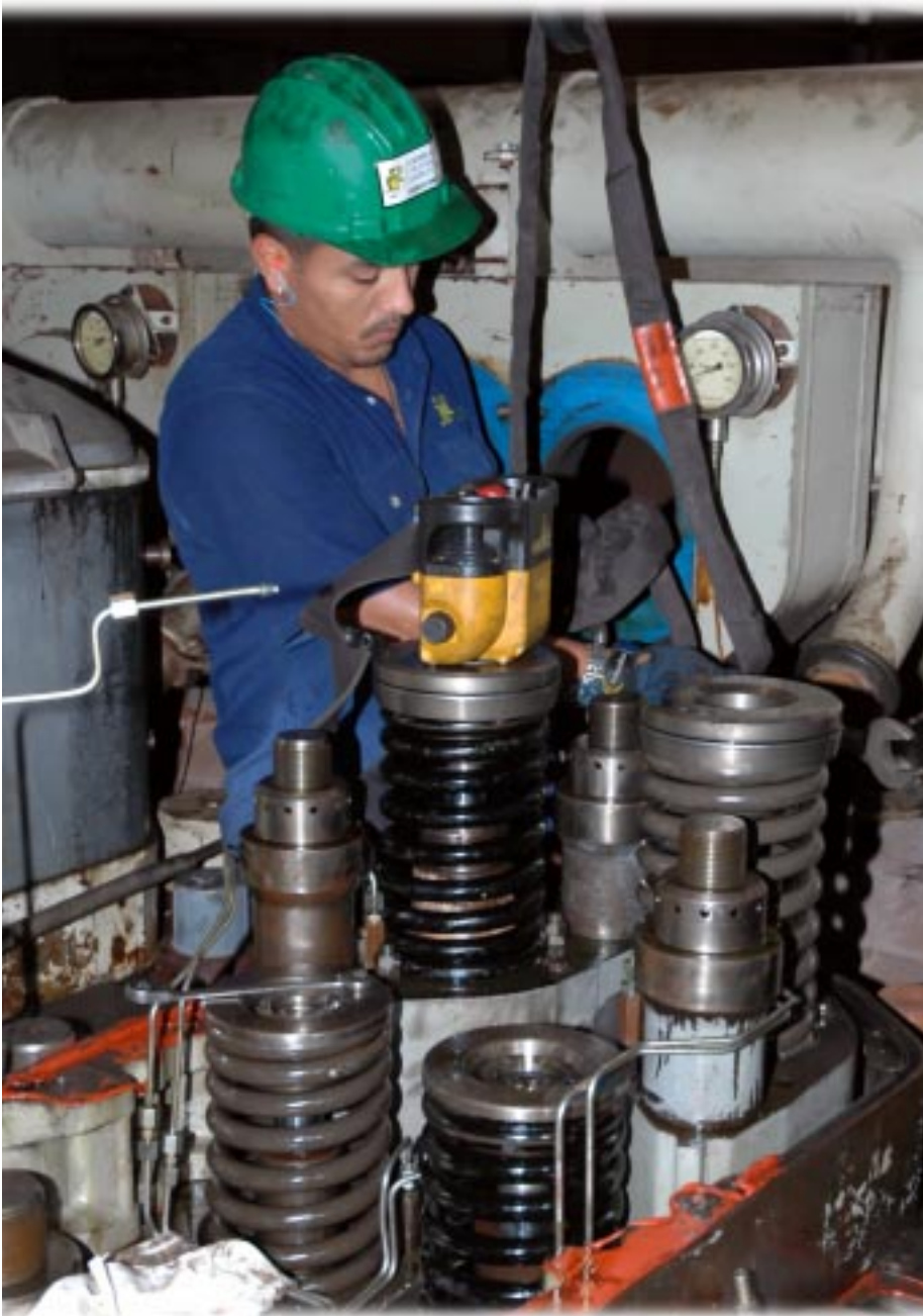
The North Sound Road Power Plant experienced major flooding during the hurricane. Damaged generators and related equipment were repaired to ensure sufficient capacity was made available for the reconnection process.
