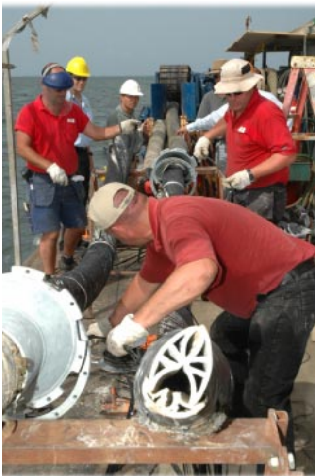
In July 2005, ABB Sweden completed repairs to the high-voltage submarine cable linking the Company's North Sound Road Plant with Rum Point which was damaged during Hurricane Ivan.
