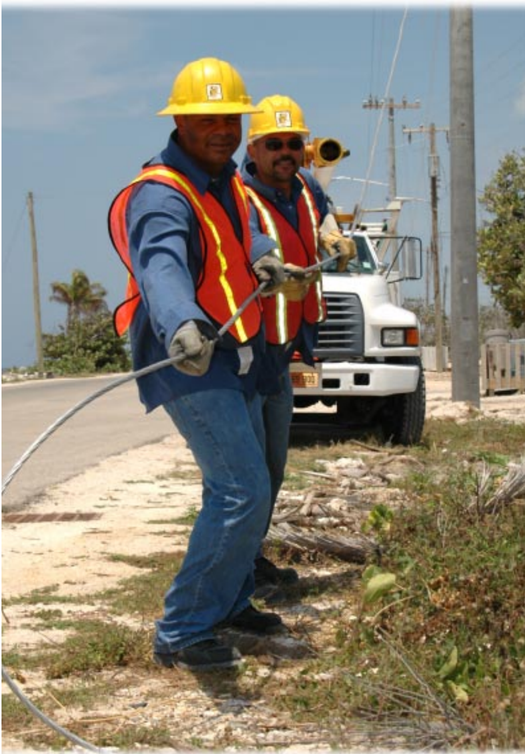
As with most employees, crews from Line Operations continuously worked long hours for weeks following the hurricane, completing major transmission and distribution system reconstruction and service connections.
