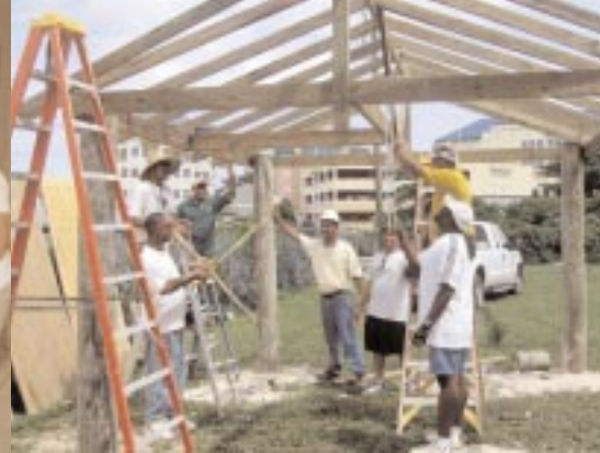
Spending Saturday mornings with other employees can be quite enjoyable and rewarding, especially when it is spent constructing a much-needed cabana on the field at Truth For Youth School. Members of the Line Crew spearheaded the project with support from other employee volunteers. Budding contractors included Kary Blythe, Dave Thompson, Gary Whittaker, Gerry Holness, Greg McLaughlin, Jessie Bodden and Michael Whittaker.
