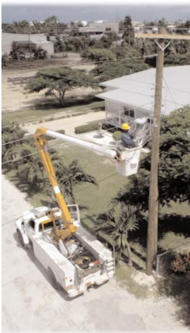
Our dedicated team of linemen help to ensure that our over 21,000 customers are provided with a safe and reliable supply of electricity. Our customer base has returned to pre-Hurricane Ivan levels, and we expect to exceed the pre-Ivan peak demand of 85 MW this summer.
