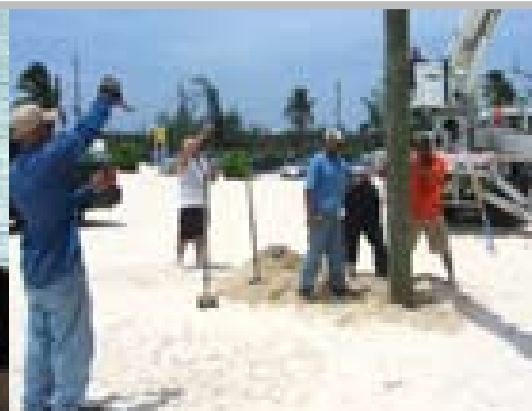
Lining up the installation for one of the 66 poles planted for the rebuilding of the 10 new cabanas at the Seven Mile Public Beach are volunteers from CUC and MasTec Inc., our line subcontractors, who partnered with us to carry out this major restoration project in 2006.
