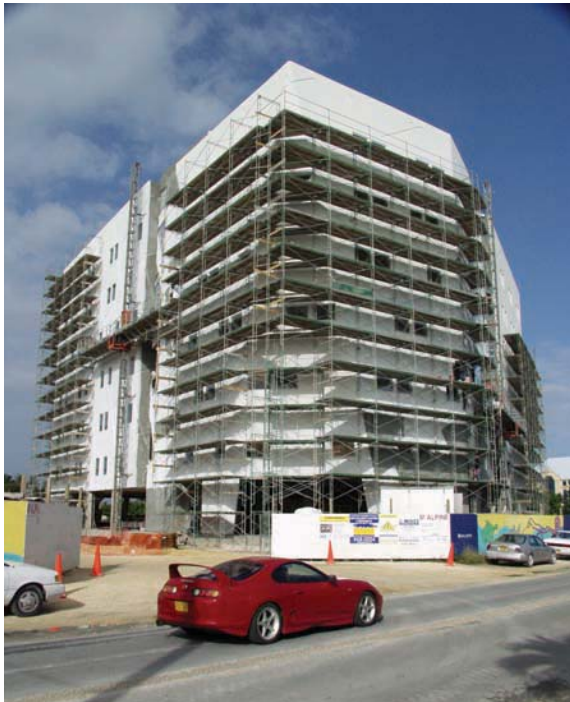
Construction on the 100,000 square-foot Walkers Building in the George Town area is ongoing as the private sector continues to invest in the infrastructural development of Grand Cayman.
