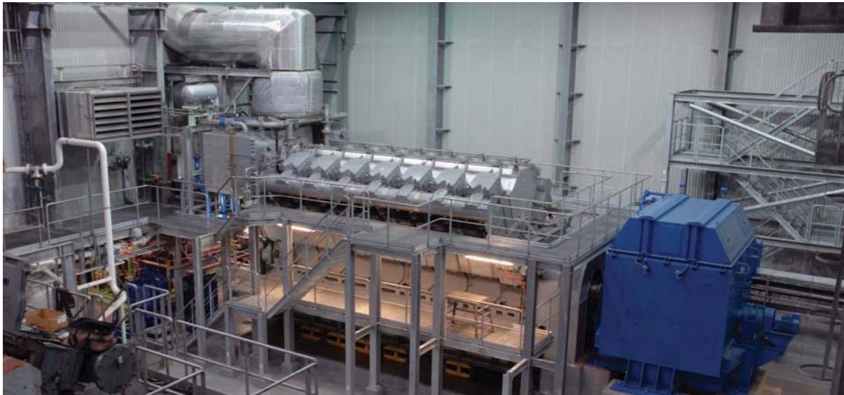
The Company's largest engine room currently houses three 12.5 MW MAN Diesel SE units and our latest addition, a MAN Diesel SE 16 MW unit, which was installed and commissioned in June 2007.
