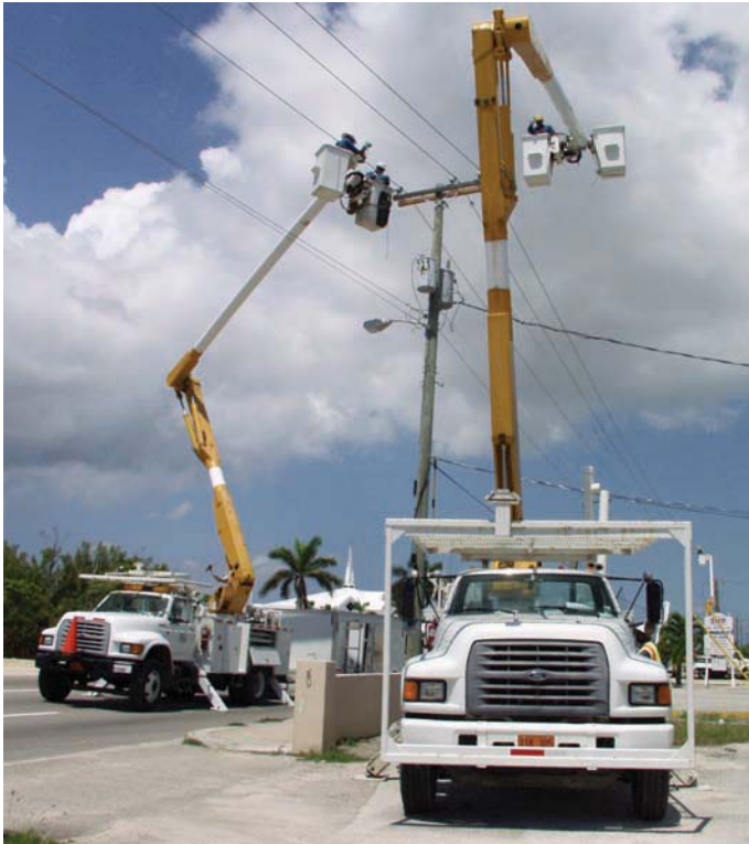
CUC's linemen and other employees endure hours of working in the unforgiving sun and heat associated with a tropical island. Their professionalism, dedication and commitment to ensuring projects are completed within schedule and to the highest standard are a testament to their character.
