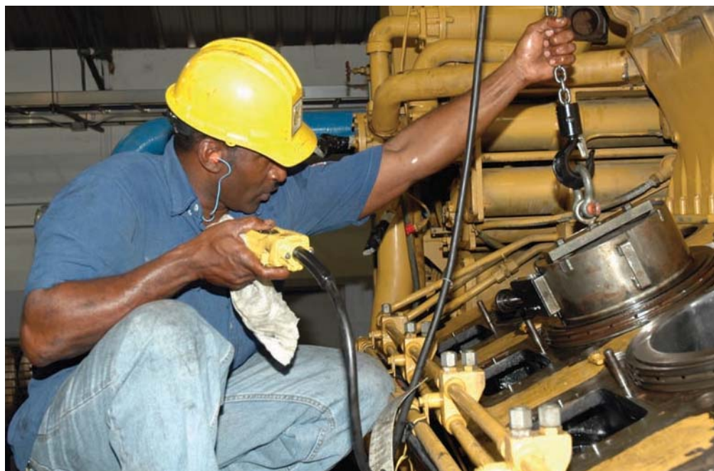
The Company's generating units undergo a thorough maintenance schedule to meet production requirements and ensure maximum efficiency.
