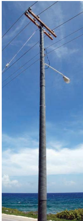
The Company began a pilot programme to test fibreglass distribution poles. Twenty-three poles were installed on a stretch of road in the East End district in close proximity to the sea to further test durability against salt spray.
