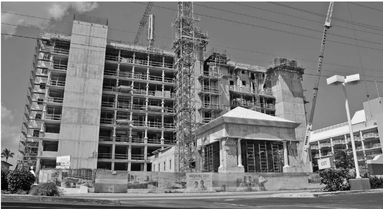
Construction continues on the Island's famous Seven Mile Beach as The WaterColours project takes shape. The Island's first nine-storey condominium complex consists of 39 luxury residences available in three and four bedroom units. The WaterColours is set for completion in 2013.
