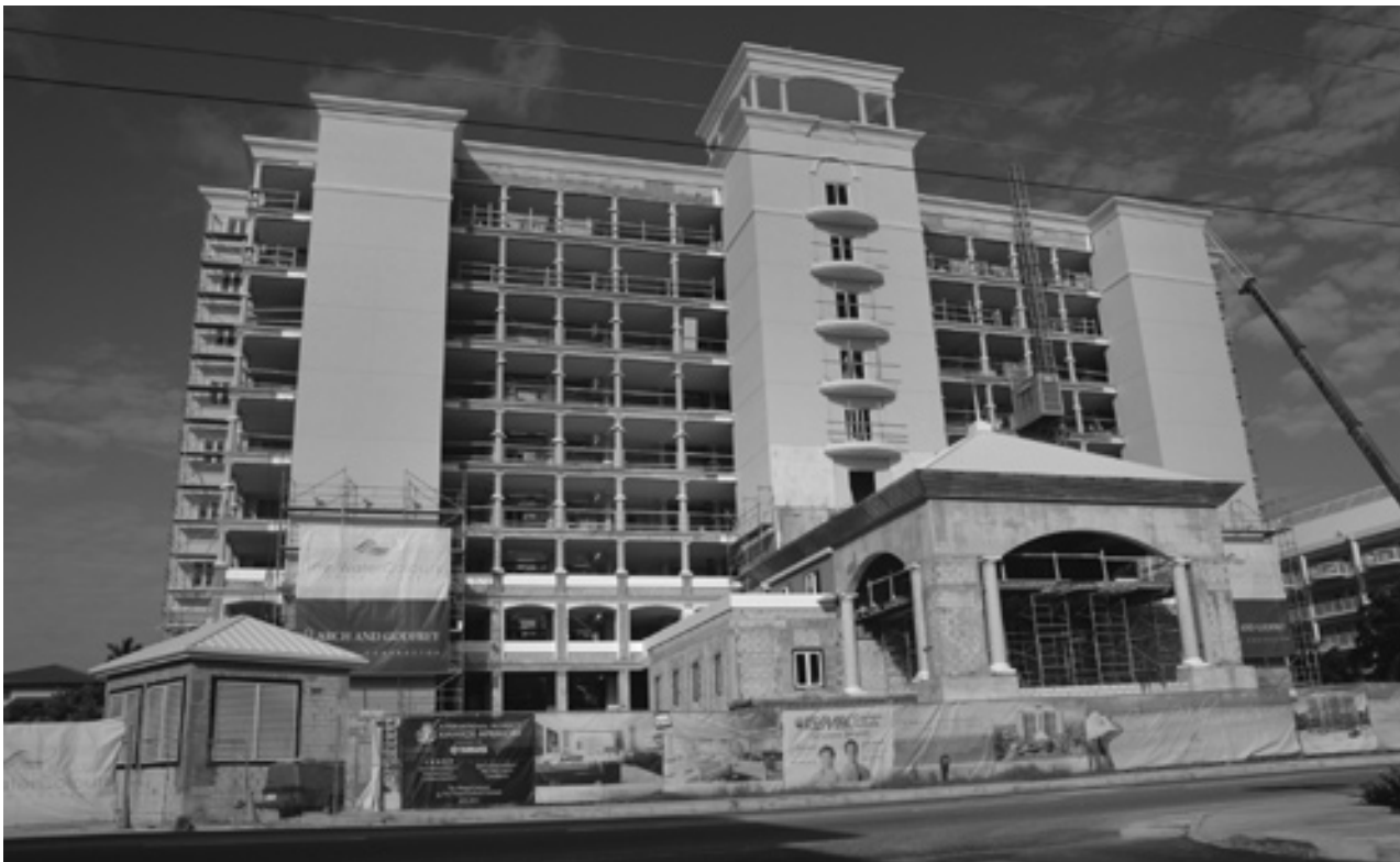
Construction continues on the Island's Seven Mile Beach as The WaterColours project takes shape. The Island's first nine-storey condominium complex consists of 60 spacious private residences available in three and four bedroom units. The WaterColours is set for completion in 2014.
