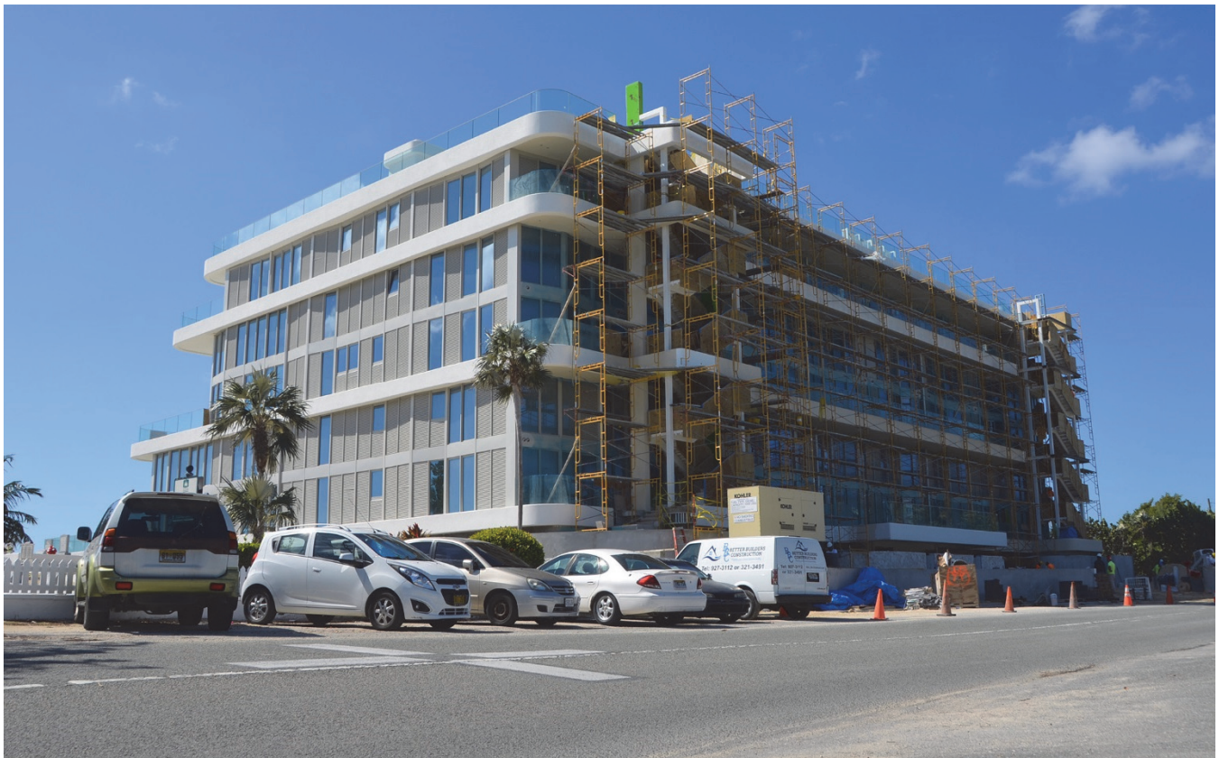
The Tides development in South Sound is one of the large projects under construction in Grand Cayman.
