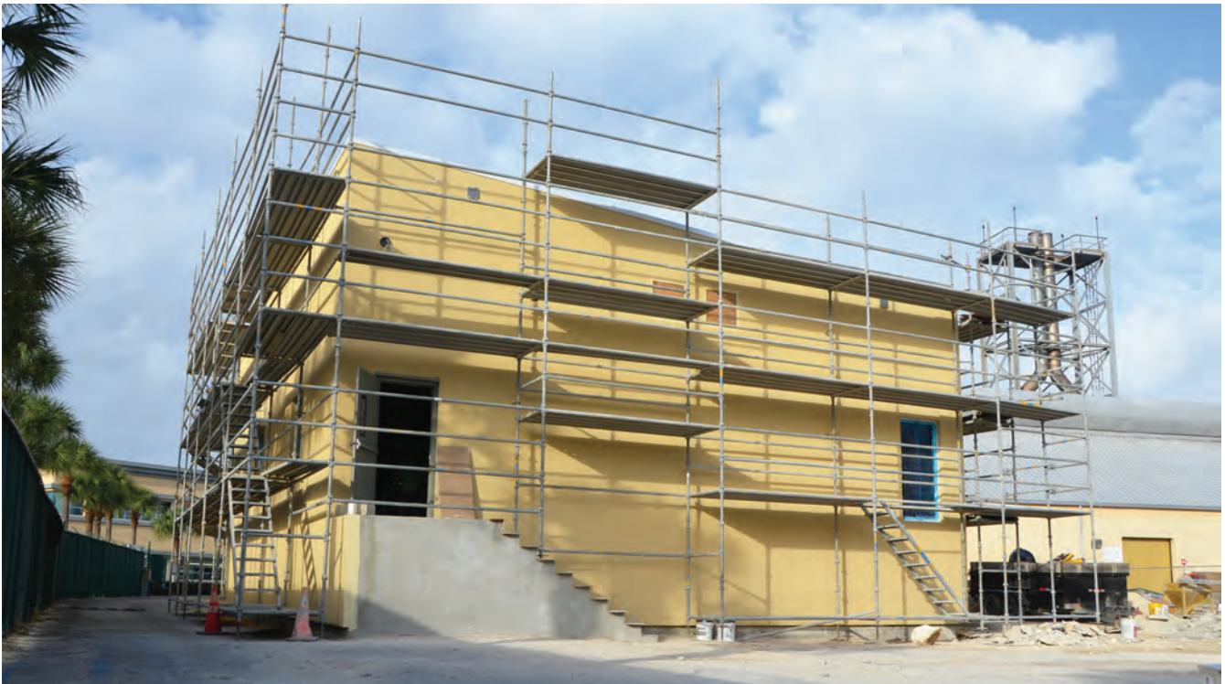
An extension to the Company's Central Control Room will be completed in 2020.
