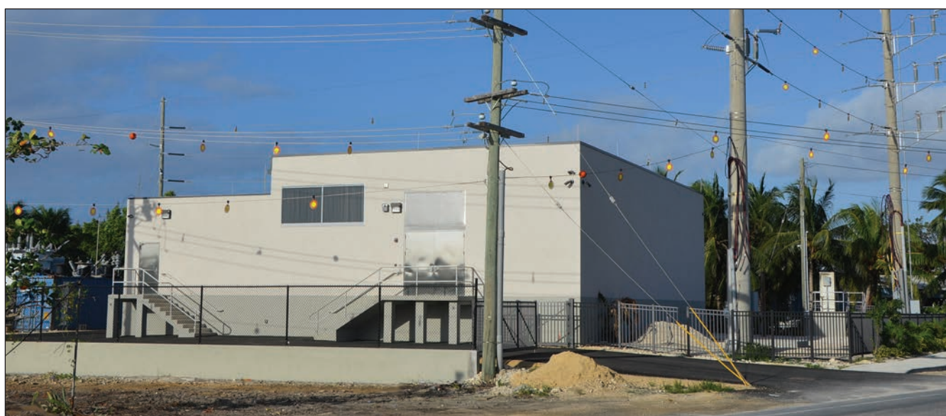
The Prospect Substation is expected to be commissioned in 2021.
