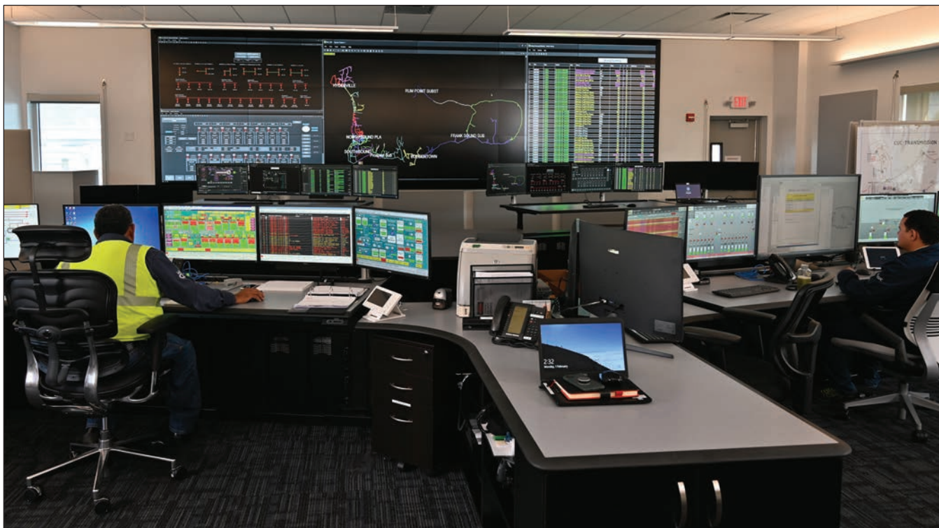
The Company's upgraded Control Room in the newly constructed Technology Centre.
