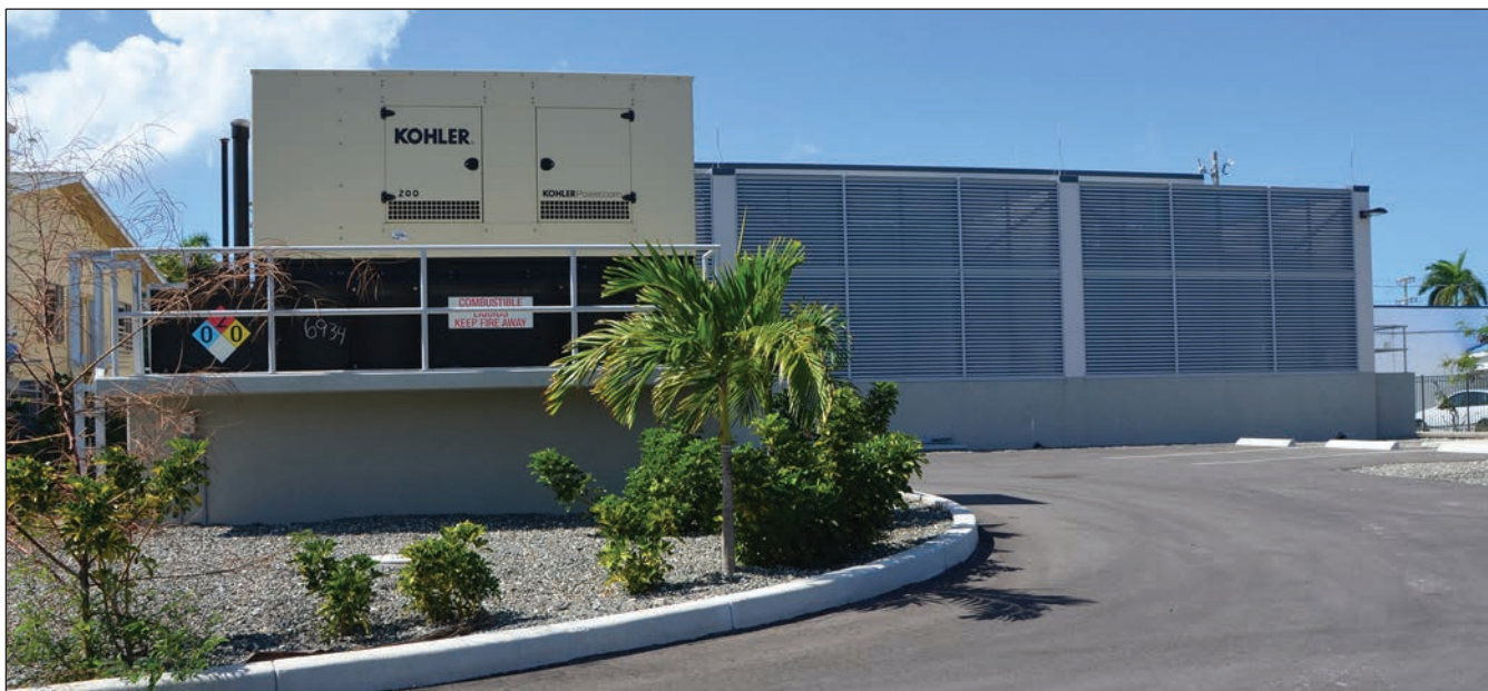
The Seven Mile Beach Substation on West Bay Road is expected to be commissioned in 2021.
