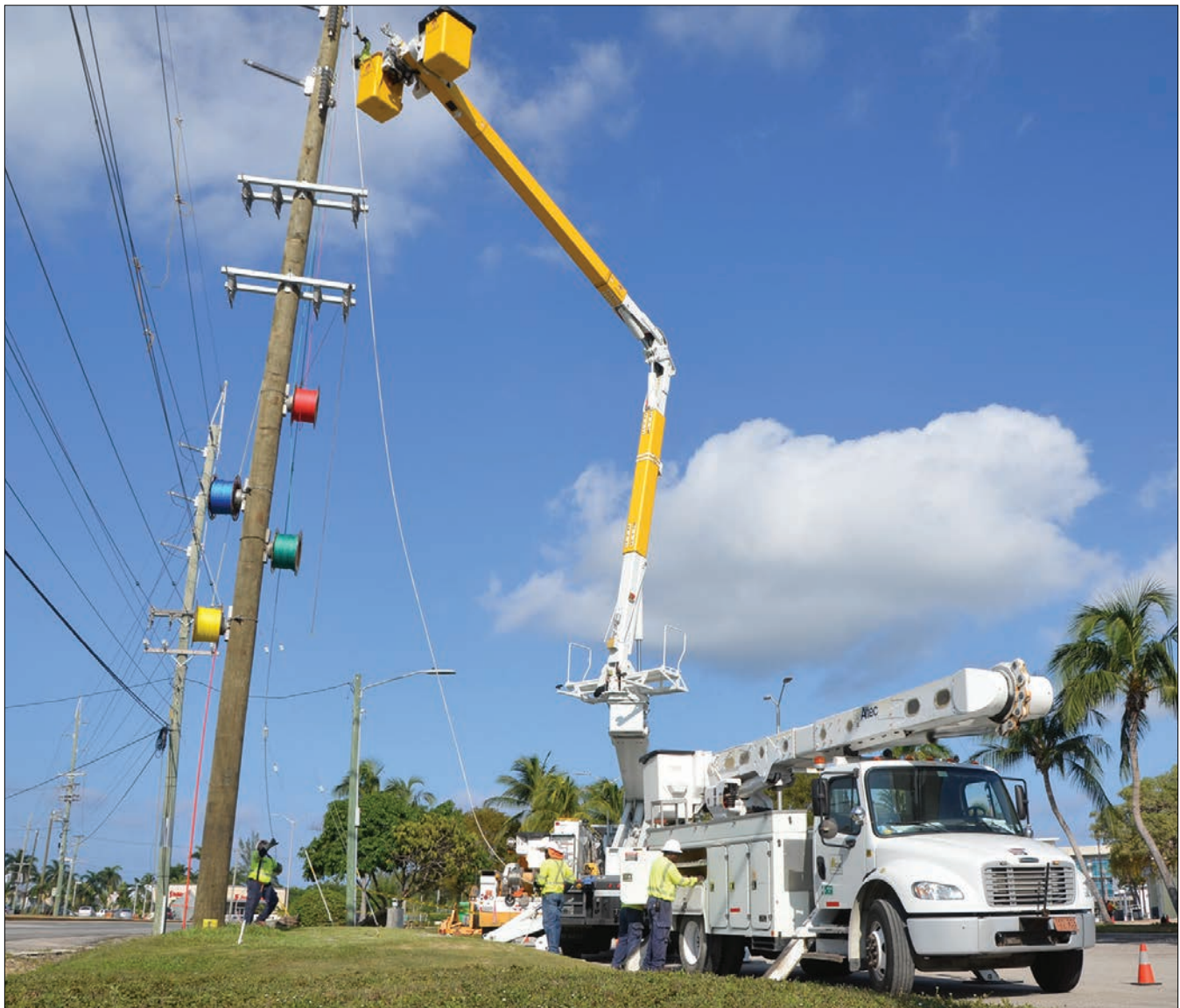
A number of major upgrades to the Company’s transmission and distribution system were carried out in 2021 to accommodate new residential and commercial customers.
