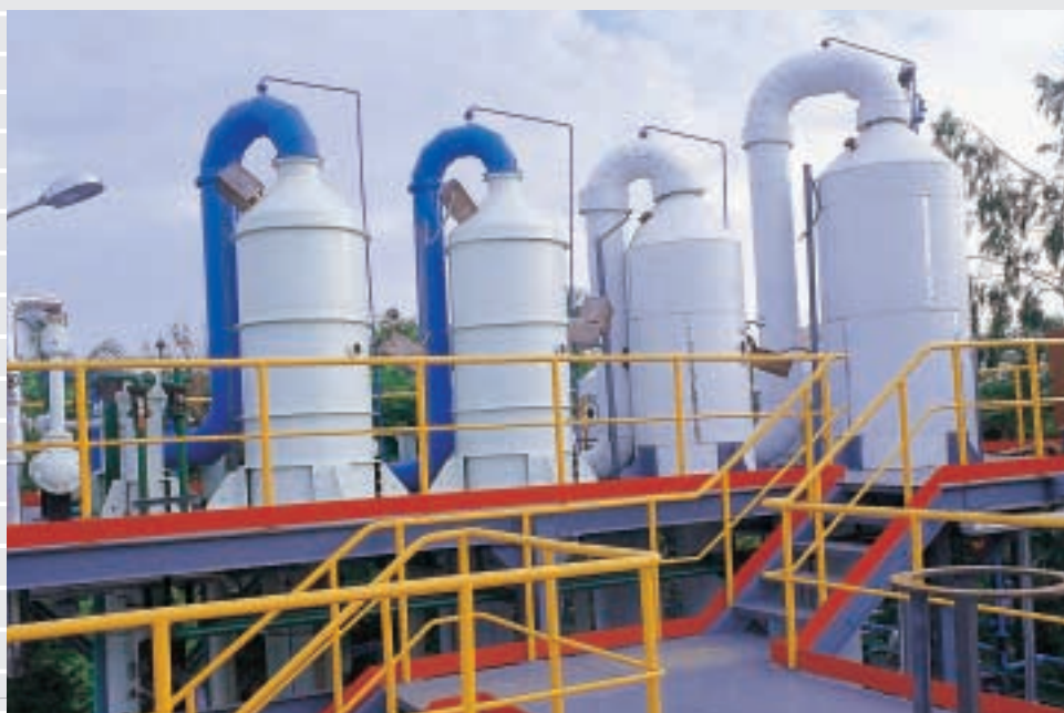
ZERO DISCHARGE facility at Bulk unit
