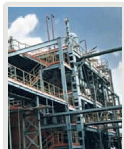
ZERO LIQUID DISCHARGE (ZLD) UNIT AT CTO FACILITY IN BOLLARAM, HYDERABAD, INDIA.
