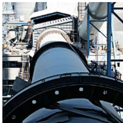
Installation of FLSmidth cement mill with Filtax filters (left) and cement kiln (right).
