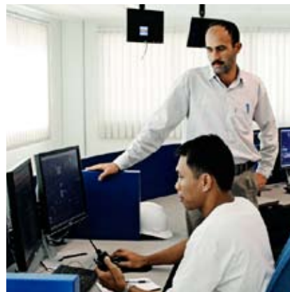
An FLSmidth Automation ECS control centre works round the clock at more than 500 cement plants worldwide.
