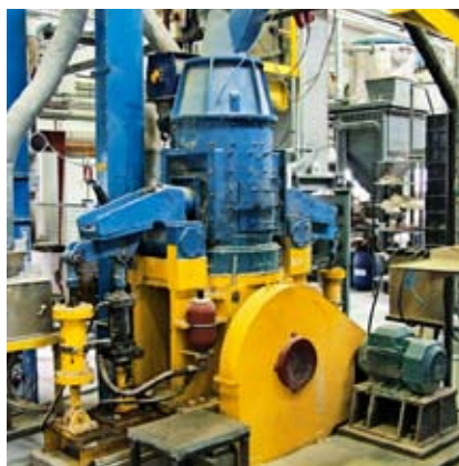
FLSmidth pilot plant for cement grinding.
