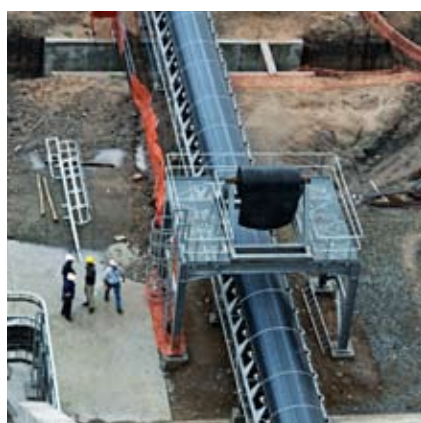
Materials handling is another of FLSmidth's core competencies. Pictured here a conveyor and a pumping station.
