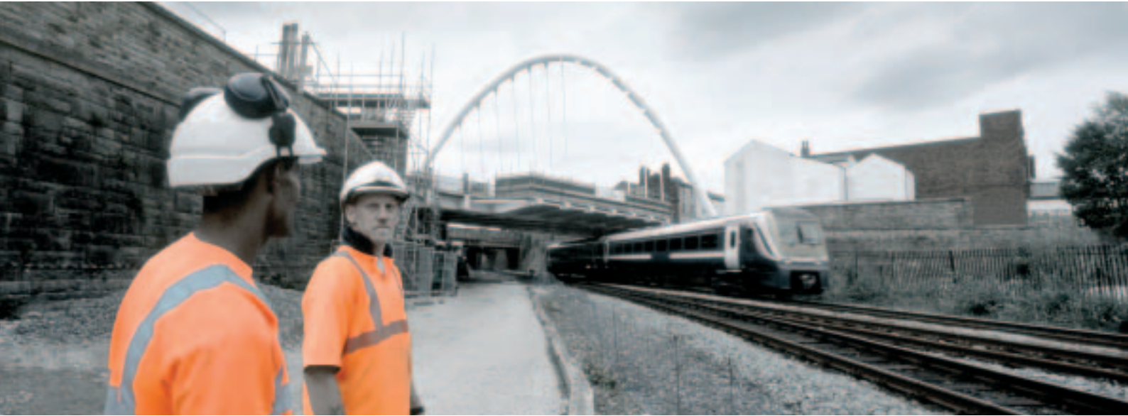
Working for Network Rail, Galliford Try Construction replaced the existing structure with a new bridge over the railway in the centre of Bolton.
