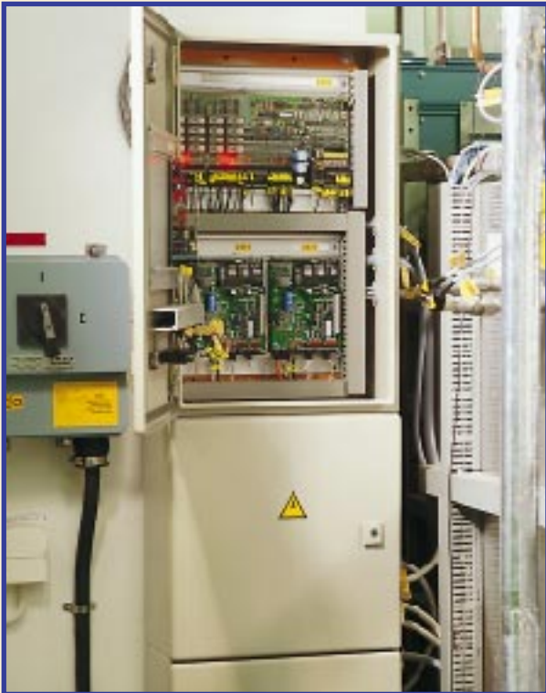
Easily accessible control unit.
