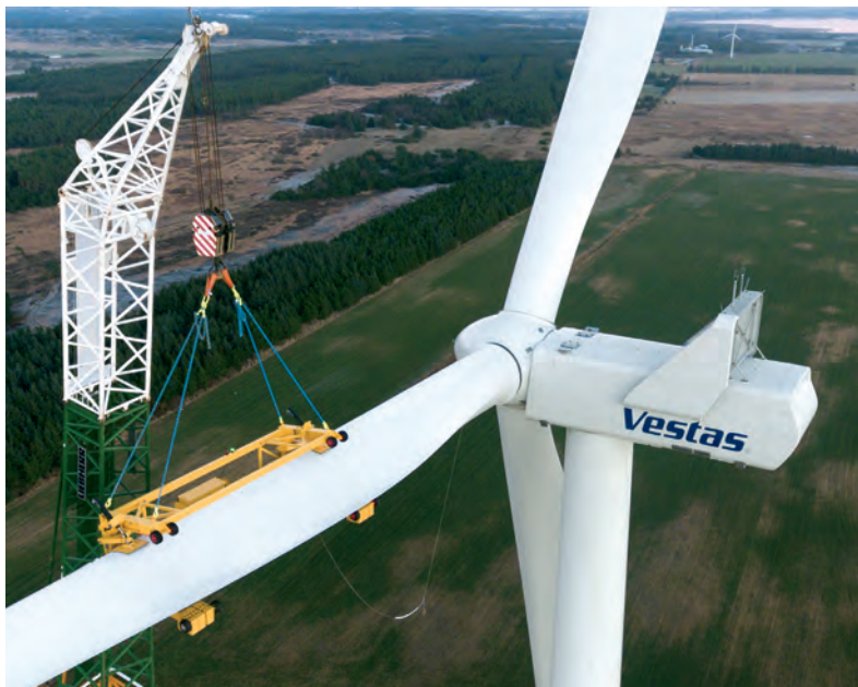
Photo courtesy of Vestas Wind Systems A/S
