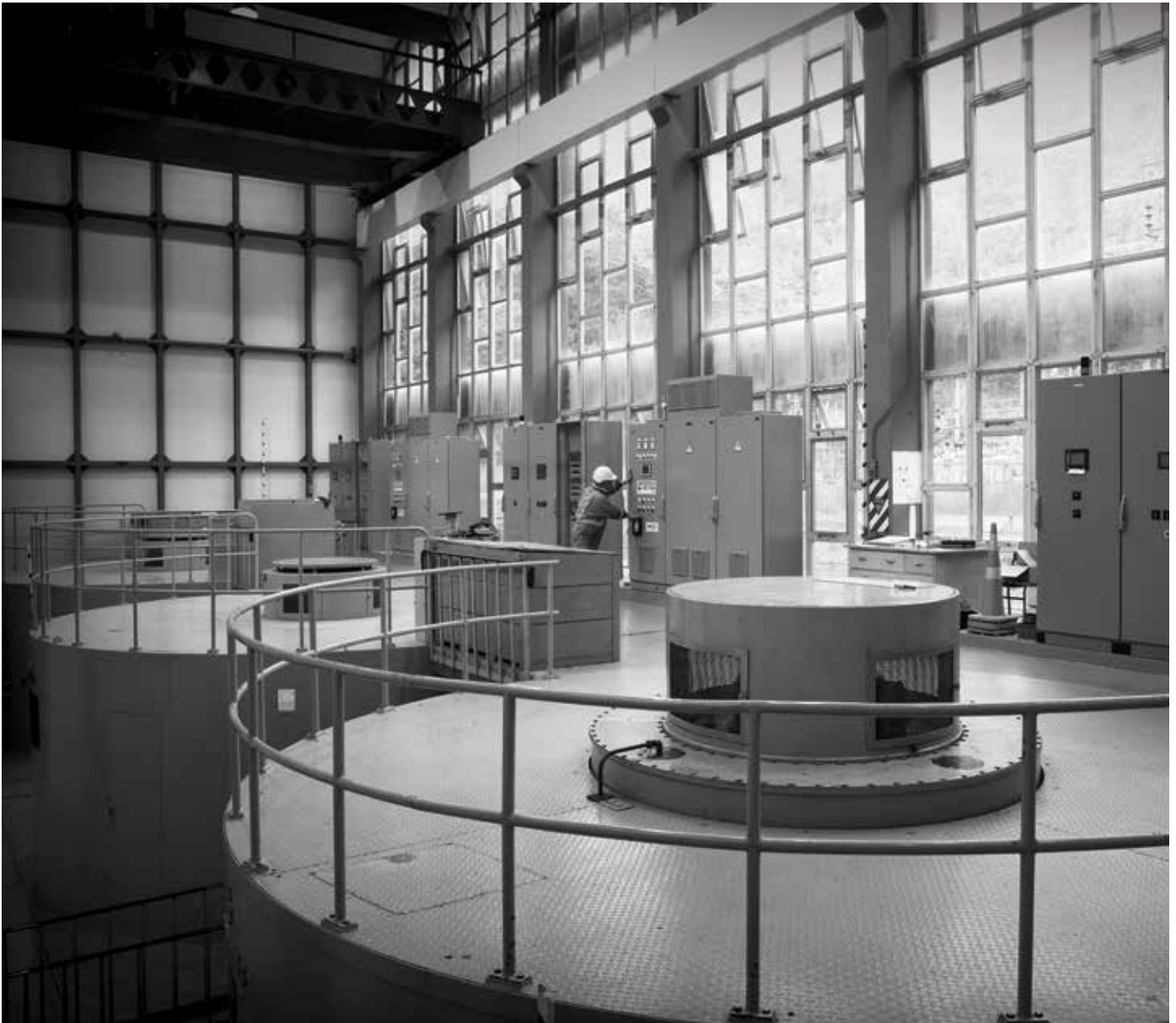
Waipori Power Station.
