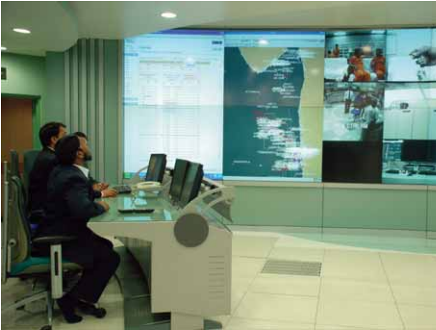
L&T's Control & Automation systems reflect the growing convergence of electrical, communication and automation technologies.
