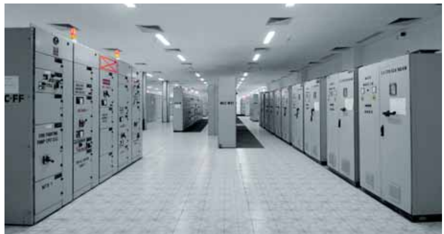
L&T's custom-designed low and medium voltage switchgear has been widely installed in industries around the world.
