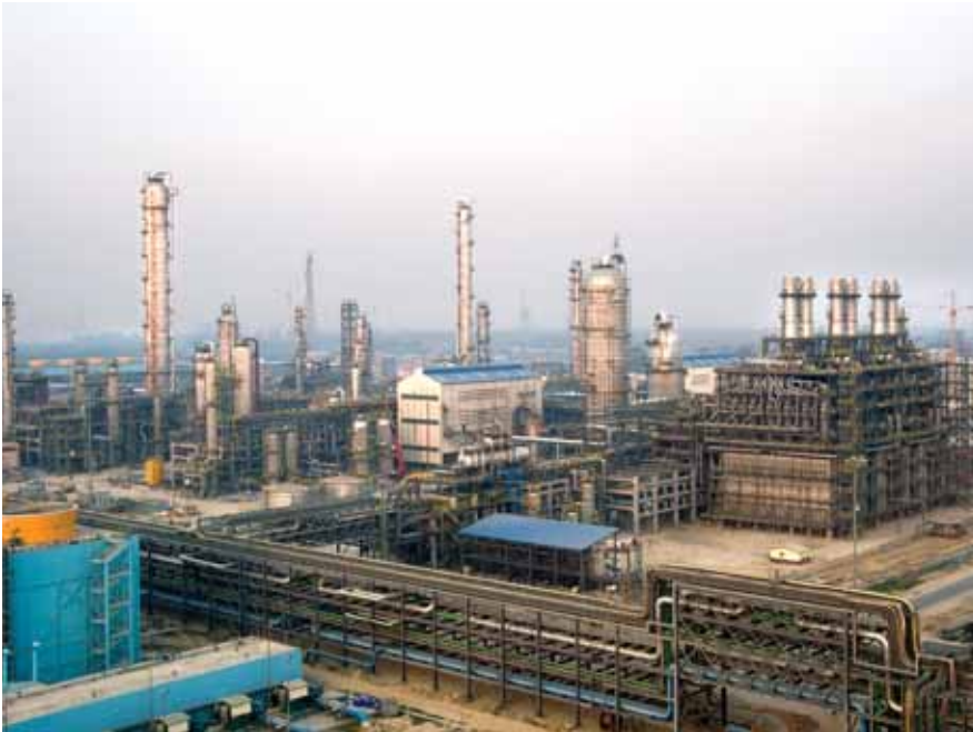
Cracking furnaces and associated units for IOCL at Panipat Naphtha Cracker Project. L&T executed this project in consortium with Toyo Engineering, Japan.
