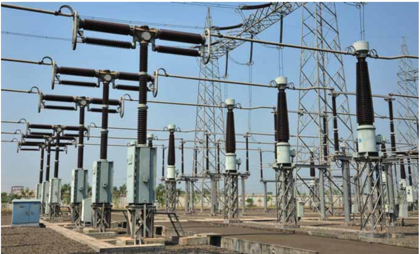
400 kV switchyard at a power plant. L&T has executed a host of such projects in India and in GCC countries. Capabilities cover design, survey, manufacture, supply, erection, testing and commissioning of switchyards and transmission lines for power grids and utilities.
