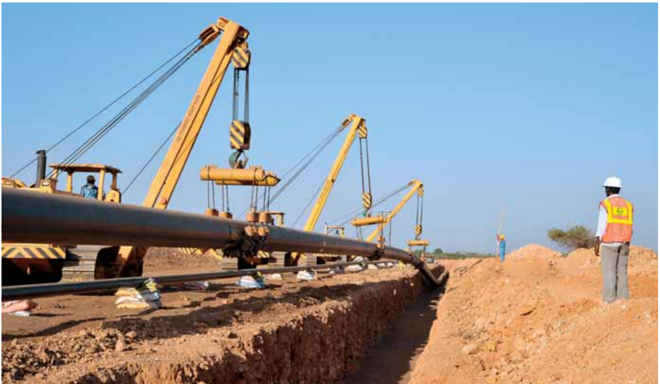
Laying of 592-km, 24" PUF-insulated crude oil pipeline along with 8" gas pipeline from Barmer to Salaya for Cairn Energy.
