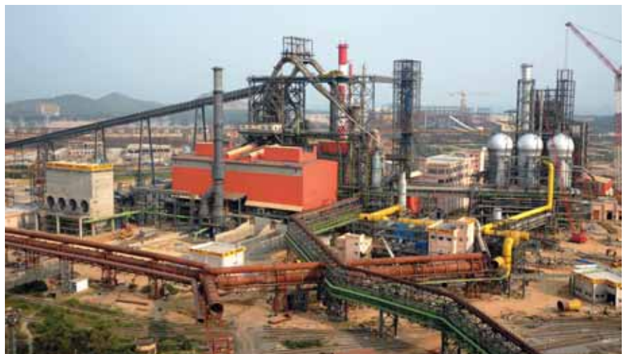
Vizag Steel Plant. L&T carries out engineering, procurement, manufacture, supply, construction and commissioning of projects in ferrous and non-ferrous metals, mineral beneficiation and coal washeries
