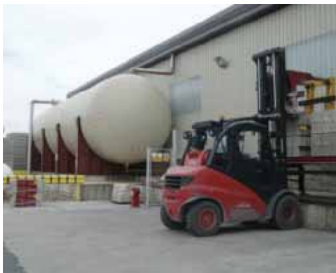
Ramsbottom Rain Water Harvesting
