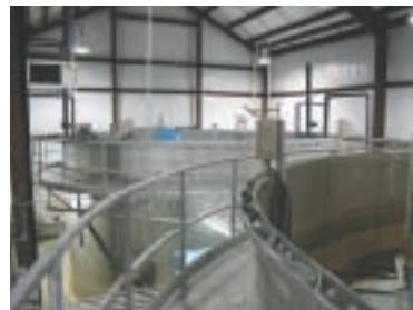
An example of a sequential batch reactor tank operating in Delaware which processes 51,000 gallons of wastewater per day.
