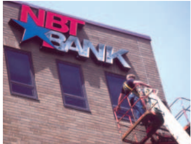
The NBT Bank sign is raised to the top of the six-floor Albany building that houses the bank’s Capital Region Financial Center. This center, located on the building’s first floor, opened in May 2004. Last year, the bank also opened two offices in the Greater Binghamton area — downtown Binghamton (July) and Endicott (September).
