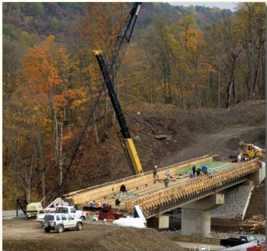
This railway bridge being constructed at Clarksburg, Pa., provides a more direct connection to the Keystone Generating Station, shown above left.
