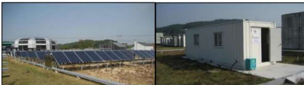
Figure 4 20kw solar PV integrated with two 25kW V-KOR batteries and the electrical grid in the field test site at Seosan-si in Korea
