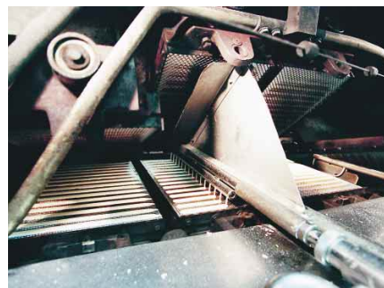
The baking ovens at the Göteborgs Kex biscuit plant in Sweden are equipped with SKF's High Temperature Bearings.
