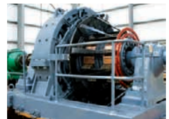
Power & Industrial's service skills have seen them extend their geographic reach with a multi-million dollar contract on a natural gas platform in the South China Sea.
