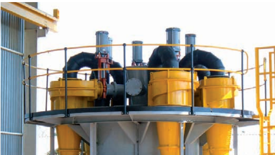
Cavex® hydrocyclones - part of the mill circuit at Waihi
