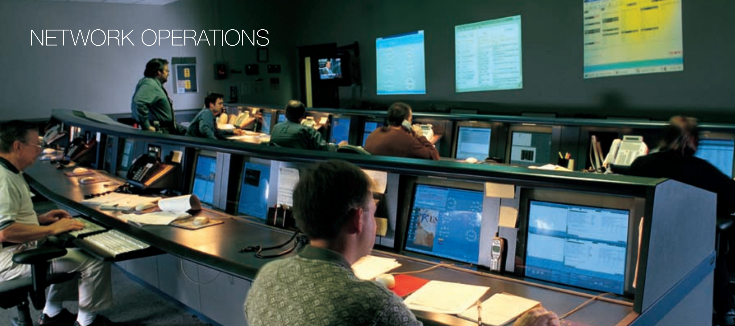
Associates in the Network Operations Center in Knoxville, Tenn., use state-of-the-art technology to constantly monitor the quality of our network.
