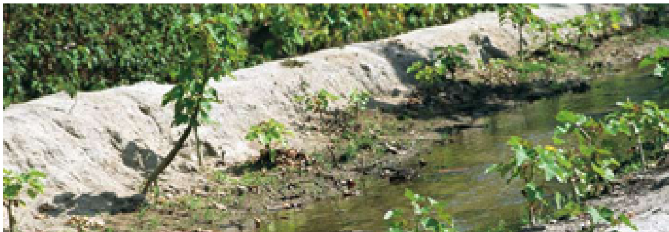
The 20 metre long water channel linking the check dam to 21 acres of farm land at BALCO and the embankment is also the venue for the plantation of 30,000 Jatrophas
