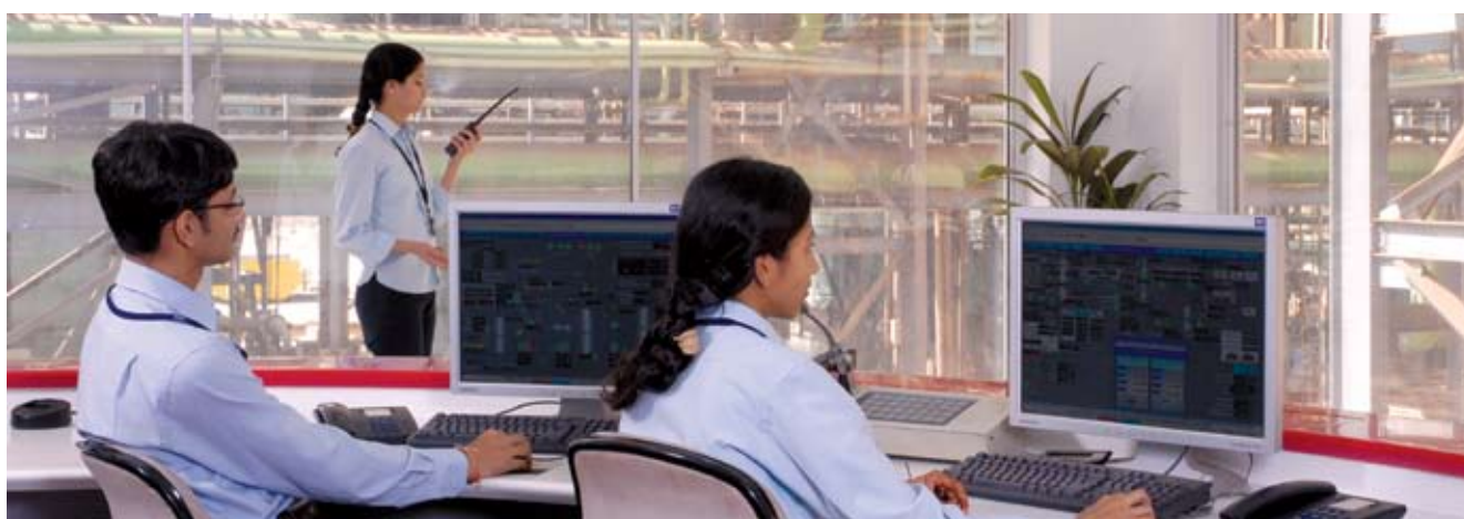
Leaching plant control room at the Chanderiya complex
