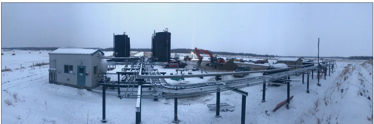
Figure 5 - Installed and commissioned upgraded Wizard Lake Facilities
