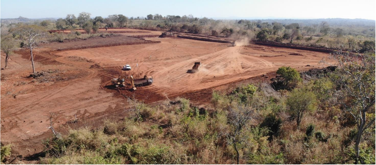
Figure 1: Topsoil removal for storage at Lindi Jumbo Graphite Project processing facility site.
