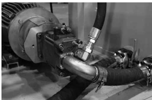
Power unit consisting of a twin (50 hp) electric motor and hydraulic pump combination, providing the power source for the "Iron Roughneck & Drawworks" on a drilling rig.
