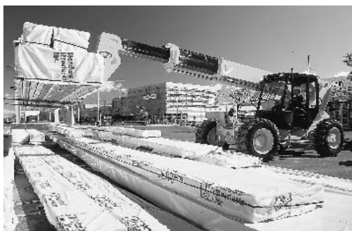
Across Canada, the construction industry moves materials with JCB products, such as this loadall telescopic handler.
