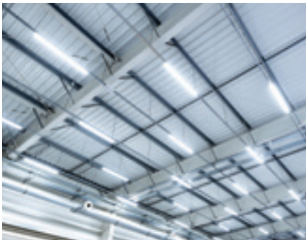
Launched Carbon Footprint Reduction Initiative with LED lighting retrofit pilot study (expected to support a ~700 tCO 2 e reduction in GHG by 2025).
