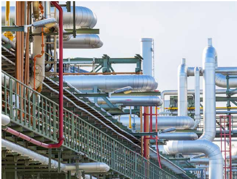
Thick sets of pipes transport raw materials, byproducts, products, steam and production-plant media exactly to where they are needed. The integrated production approach of German chemical sites has been very successful since the 1990s.
