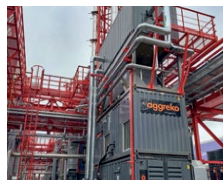
A 14 MW combined heat and power gas application for a manufacturing customer in Russia
